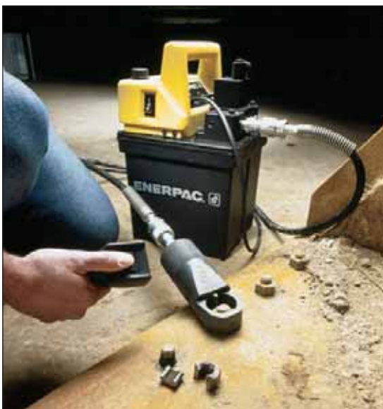
◀ This PED-1101B Submerged pump quickly and quietly powers a hydraulic nut cutter in this bucket maintenance application.
